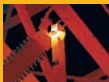
Incorrectly secured connection
