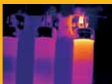
Internal fuse damage
