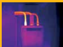
Poor connection and internal damage
