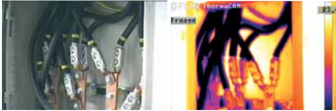
This thermal image looks quite odd, if you don't know the circumstances under which it was taken. The cables are not loaded at all. They are located in a warm room and the non-oxidized metal surfaces reflect the warm ambient temperature.
