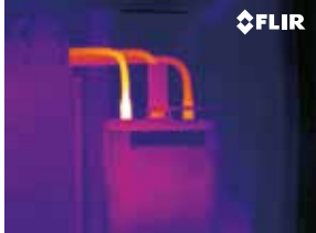
Poor connection and internal damage
