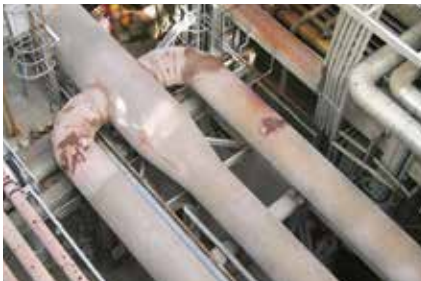
Visual and thermal image of a refractory lining breakdown in an air line.
