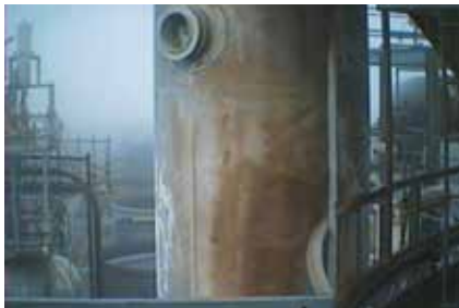
Visual and thermal image of a failure in an internal refractory lining.
