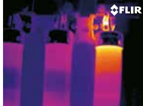
Internal fuse damage
