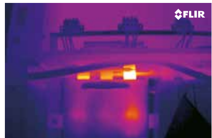
Bad electrical connection.
