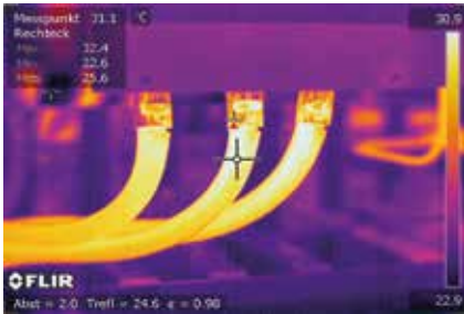
Thermal image of electrical cables.
