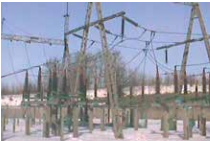
150 KV station, visual and thermal images.
