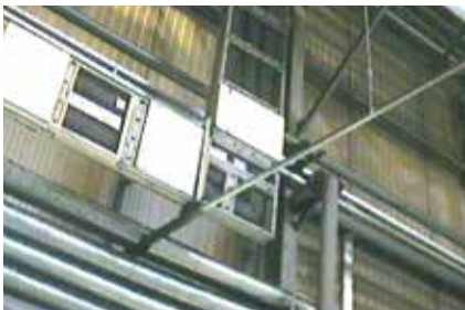
Visual and thermal image of a busbar rail system in production hall.
