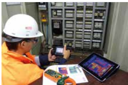
The FLIR thermal imaging camera transfers the thermal images to a tablet PC via Wireless LAN.
