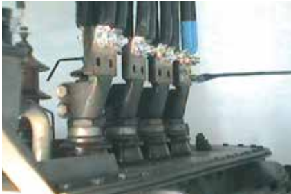
Top of transformer; high-voltage connection.
