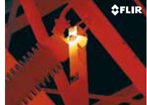
Incorrectly secured connection
