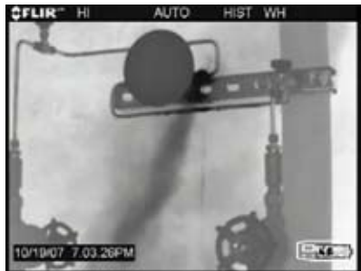
A leaking pressure gauge
