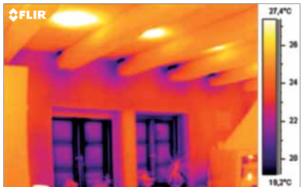
The thermal image shows thermal bridges between the roof beams and adjacent walls.
