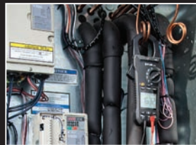
Diagnose VFD-controlled problems
