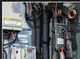
Diagnose VFD-controlled problems
